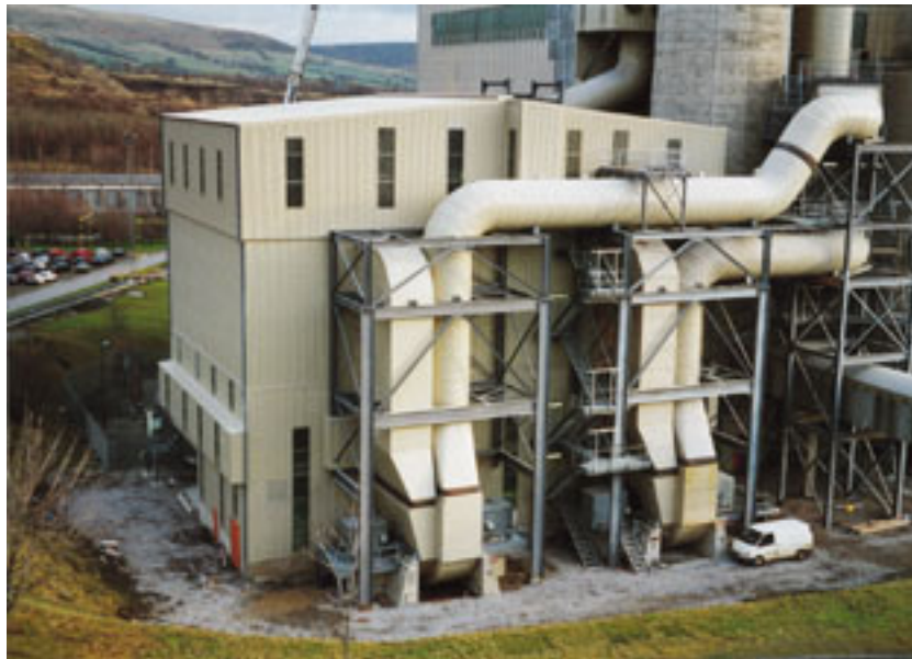
Fig 9. Cement Works Fabric Filters
