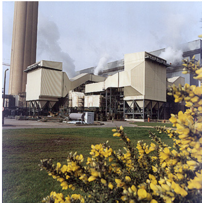
Fig 8. Additional Parallel ESPs on 4 x 500 MWe Boiler
